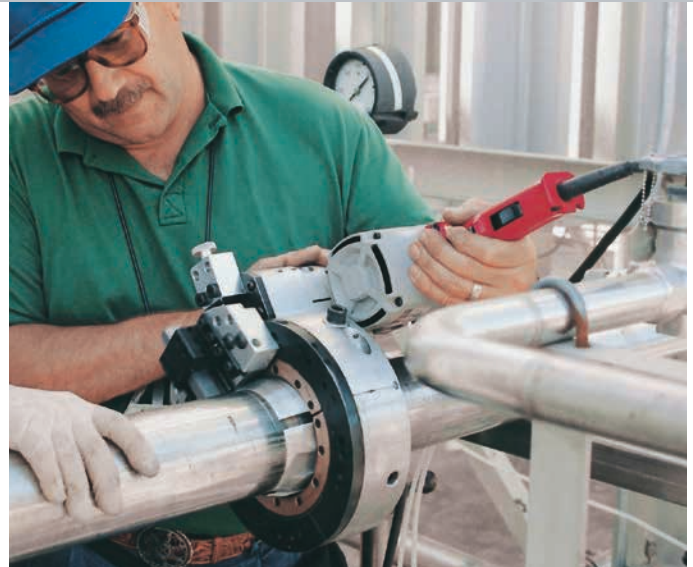
A piping system contractor performing outage maintenance on thin-wall stainless piping system uses an electrically powered SB clamshell fitted with full support pads. The piping system was part of an auxiliary high purity nitrogen supply line at a semiconductor manufacturing facility. A prefabricated pipe assembly was then orbitally welded in place without any additional end-prep being required.
