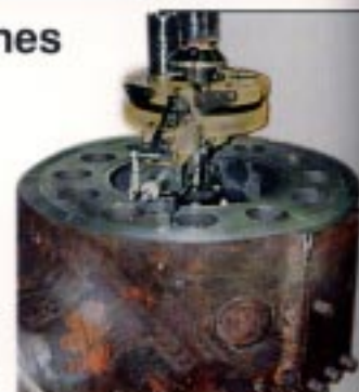
I.D. mounted EP-3 End Prep Lathe re-facing a 36" O.D. Main Steam Stop Valve.
